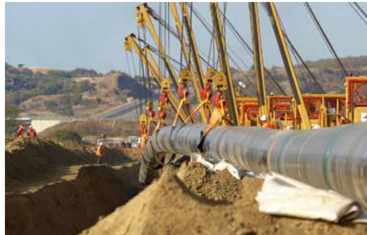
Works are ongoing to build the controversial Trans-Adriatic Pipeline, which will transport gas from the Caspian Sea to the Mediterranean at a time when more investments in renewable grids are needed. Source: TAP-AG
